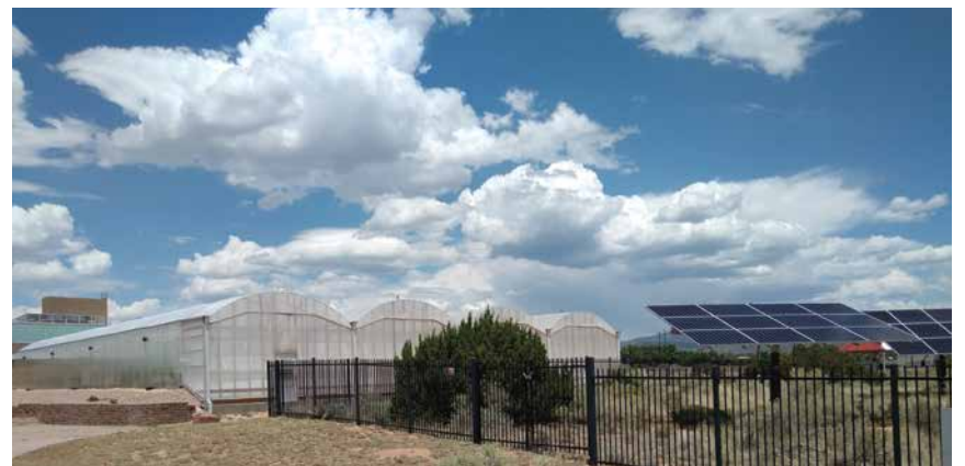
SFCC's 11kW tracking solar array provides power to the 12,000-sq.-ft. off-grid controlled-environment greenhouse.
