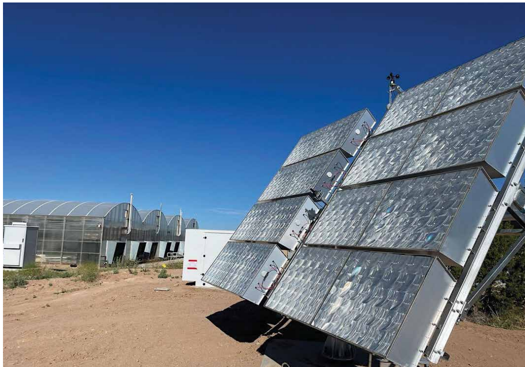
Solar cPV prototype tracker from Integrated Solar Technologies operates off-grid or with the campus educational microgrid, supporting systems in the 12,000-sq-ft. CEA greenhouse.
