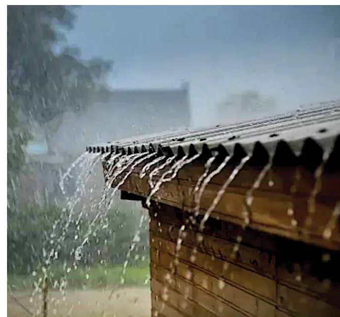
Water not being captured as it flows off a roof
