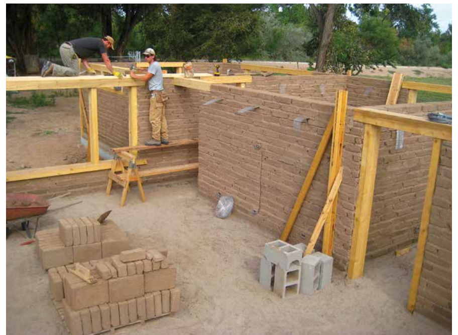
Retired contractor Pat Martínez Rutherford, of Soledad Canyon Earth Builders in Las Cruces, N.M., reveals a just-completed multi-colored rammed-earth wall. It is the focal point of an outdoor kitchen. Four different colored crusher fines were used to create the wave effect. Pictured on the far left is Soledad Canyon employee, Raul Muro.
