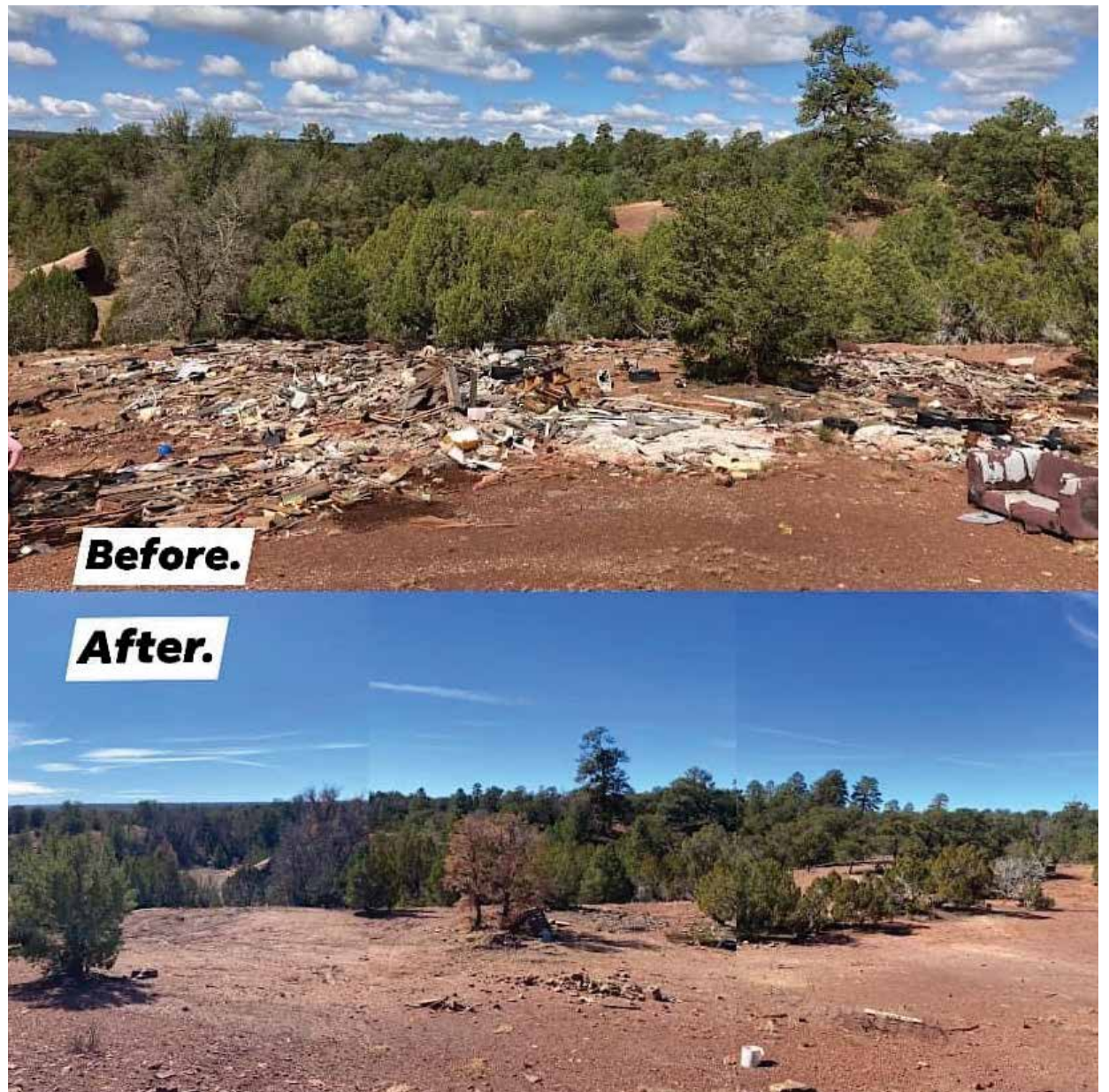
Nibi K'é Baá "Love on the Land" landfill cleanup and watershed restoration. Aside from the natural building projects we have been cleaning up illegal landfills started years ago by the first settlers (trading posts, Catholic Church and U.S. military) in our territory. After the cleanup, we planted plants that detoxify soil throughout the area. We want to relate to our homelands the way our ancestors did, and re-experience it by re-stewarding and regenerating that deep love for land and life... to regenerate kinship and culture. Photo courtesy Nibi K'é Baá
