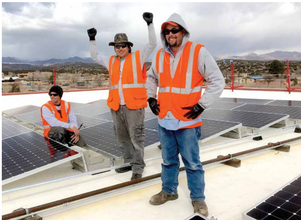
Solar installers at Cochiti Pueblo. Local Choice Energy would allow tribes to generate and sell electricity.
