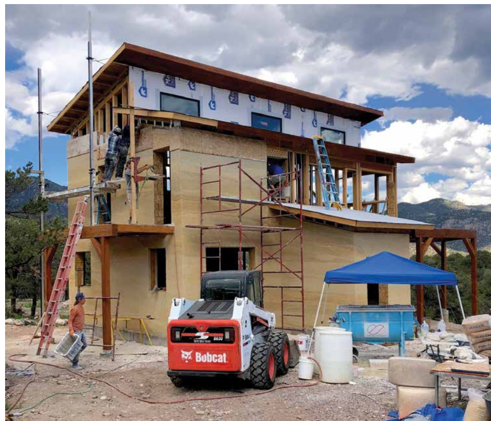
Hempcrete residential wall cast installation (in process) by the Hemp Building Company, Longmont, Colo. WWW.HEMPBUILDINGCO.COM
