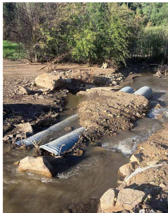
A two-culvert replacement for a three-culvert road crossing blew out shortly after replacement.
