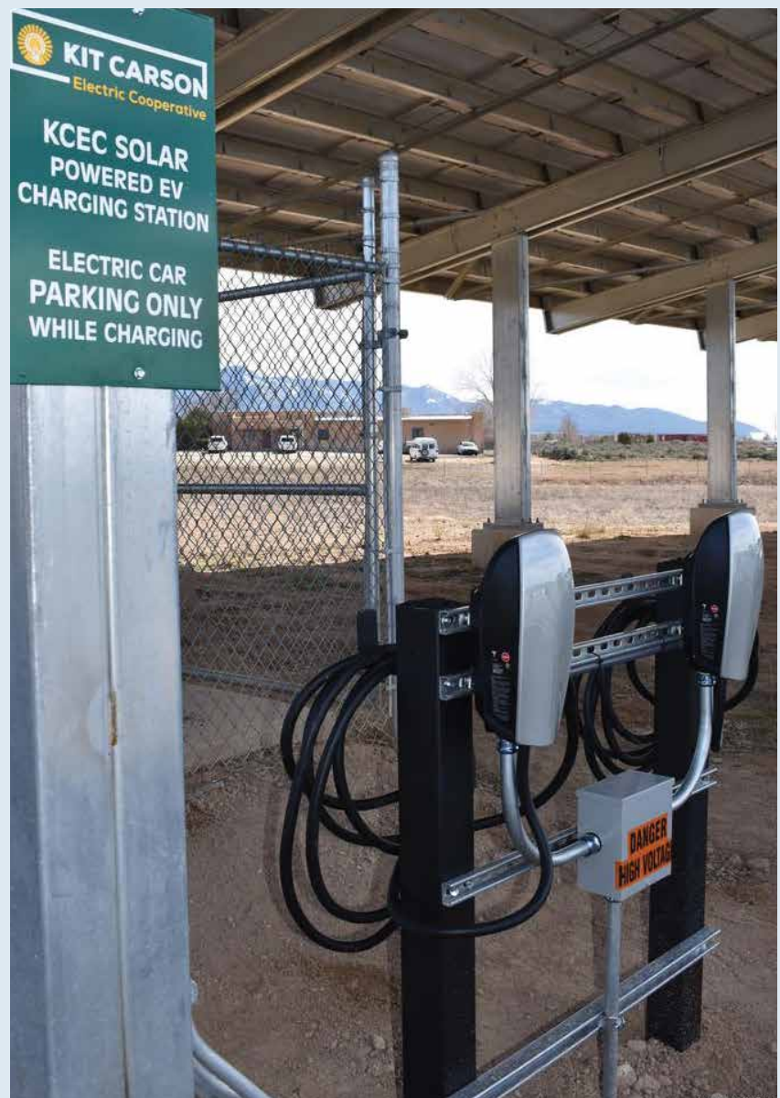
Kit Carson Electric Cooperative Electric Vehicle Charging Station
