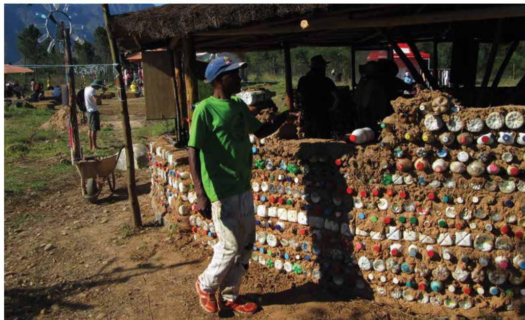
Constructing an Ecobrick round house at the dumpsite near Greyton, South Africa, 2014
