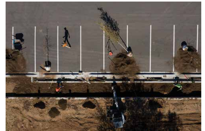
The RainCatcher crew builds a raingarden at Santa Fe High School. This system will divert stormwater from the parking lot to plantings, where it can be filtered and slowly soak into the aquifer.
