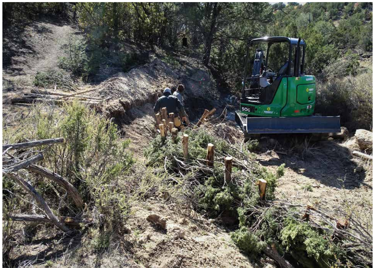
Gully stabilization with a juniper palisade below a single-tread backcountry trail in the Eldorado Community Preserve's woodlands.
