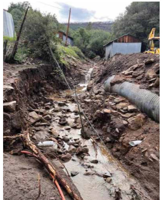
Acequias, culverts, domestic water lines, fiber-optic cables and county roads were destroyed in some communities.
